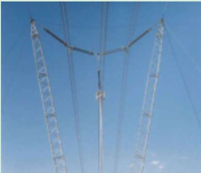
Fig. 4: Compact cross rope configuration (note centre phase is slack in this case due to tap off (not shown))
